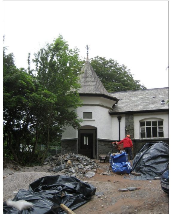
Scheme in progress in 2009 at the Reading Rooms, Coniston for Mitre Housing Association, after a CRHT survey in 2006
